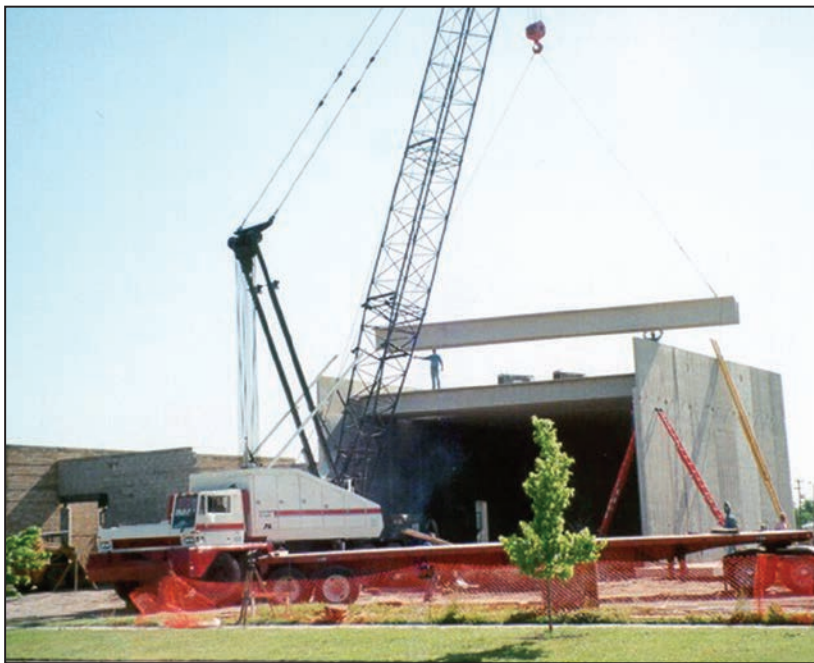
Figure A3-1. The addition to this school was designed to serve as a multi-use safe room; it is also used as a cafeteria, gym, and large-group gathering space (Wichita, KS)
