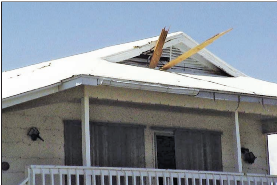
Figure B8-10. Impact of structural wood members in the gable end from a neighboring house (Pine Island, FL)
