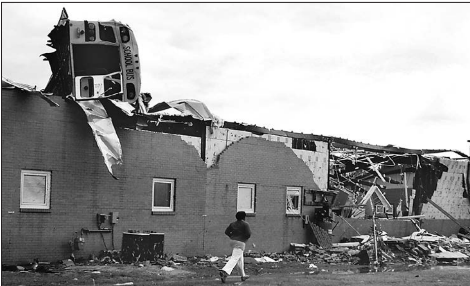
Figure B8-7. Large debris: A school bus was lifted atop a school (Caledonia, MS, tornado, 2008)
