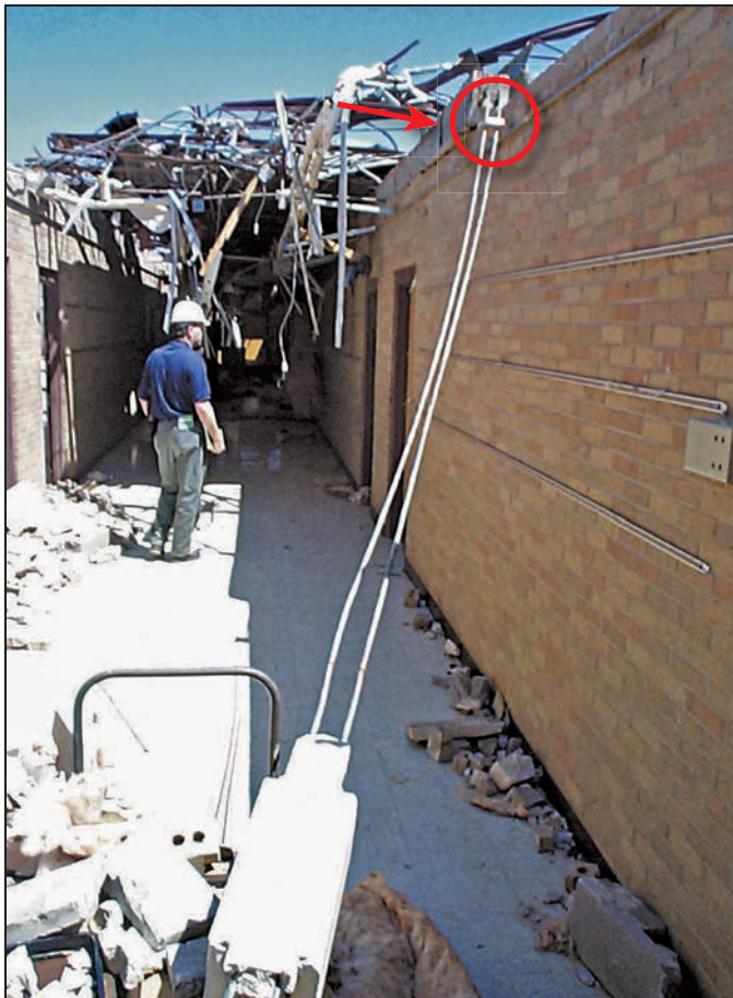
Figure B3-8. Failure of load path between the bond beam and the top of the unreinforced masonry wall when struck by an F4 tornado (Moore, OK 1999 tornado)
