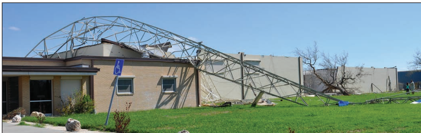
Figure B3-13. Laydown of communications tower onto a building (Rockport, TX, 2017 hurricane)
