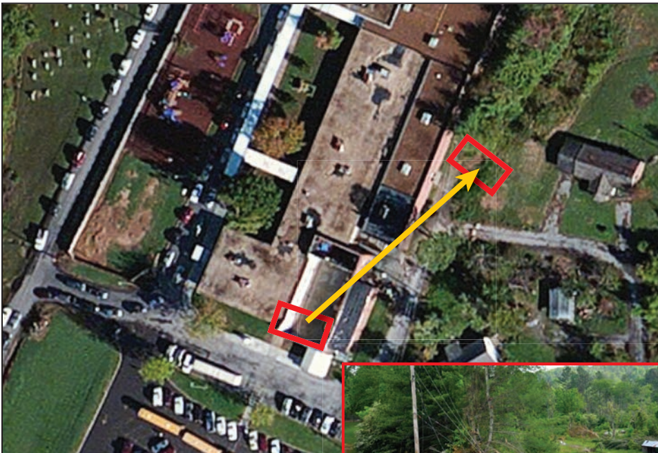
Figure B8-5. Large debris: An EF1 tornado blew a school gymnasium's steel truss and steel deck roof assembly approximately 230 feet (Cleveland, TN, 2011)
