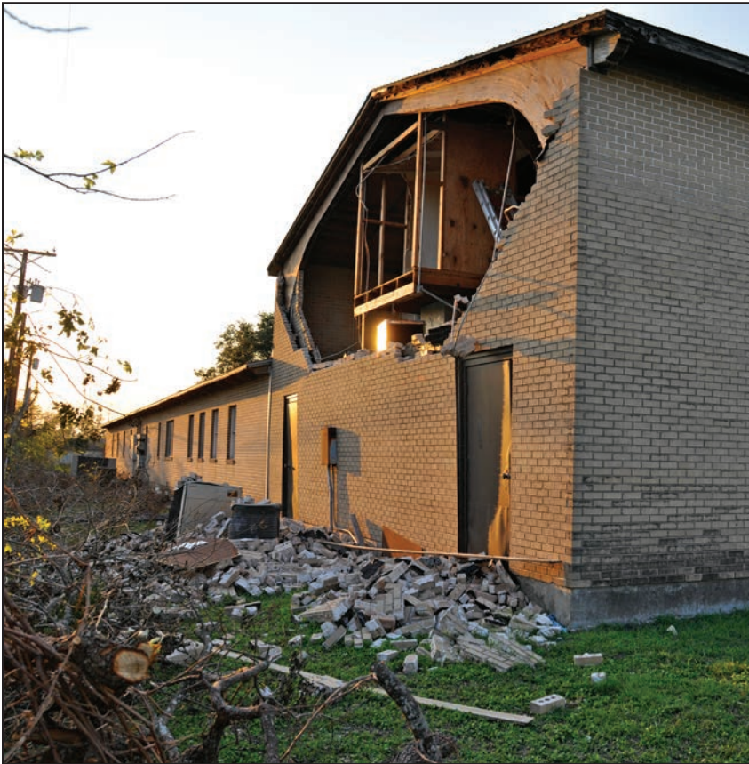
Figure B3-15. Example of falling debris impact: Brick veneer failure on church (Refugio, TX, 2017 hurricane)
