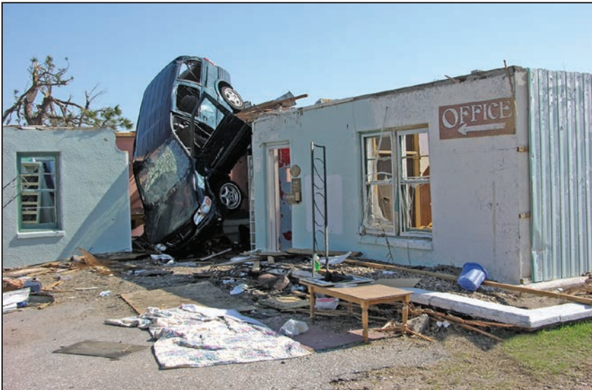
Figure B3-16. Vehicle rollover (Greensburg, KS, 2007 tornado)
