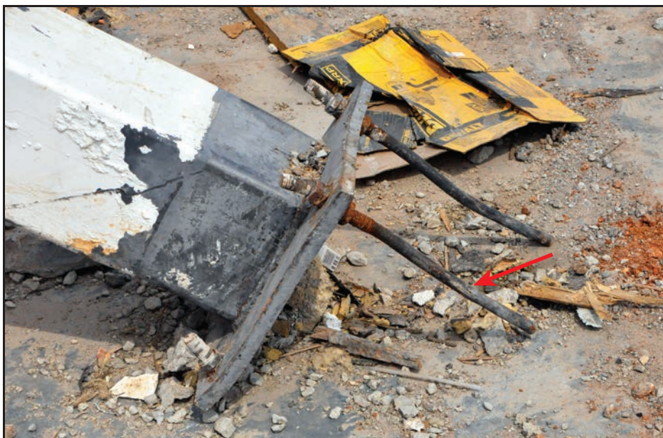
Figure B3-9. Bolt failure at interior column resulting from shear and tension. The hooked anchor bolts pulled out of the slab (red arrow) (Joplin, MO 2011 tornado)
