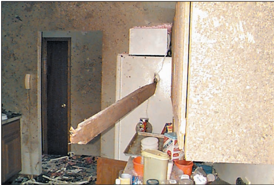
Figure B8-9. Refrigerator pierced by a 2x6. The portion of the 2x6 that is visible was 4 feet 8 inches long. It went several inches into the freezer compartment. (Oklahoma City, OK, 1999 tornado)
