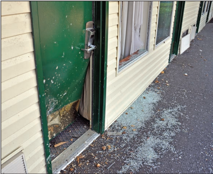
Figure B8-18. This metal door was damaged by windborne debris generated by a weak tornado. The bottom hinge was damaged, but the single latch was able to resist the modest wind and impact load. The door was on the verge of failing. (St. Louis, MO, 2013 tornado)
