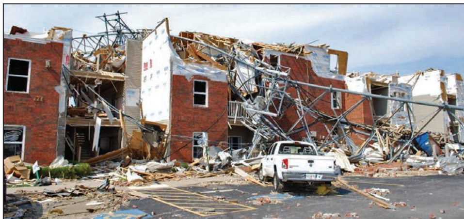
Figure B3-14. Laydown of a large communications tower onto a building (Joplin, MO, 2011 tornado)
