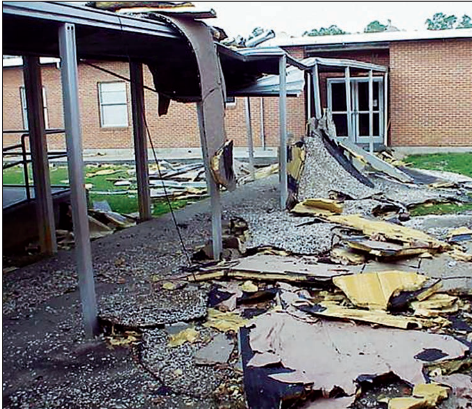
Figure B8-1. Medium debris: Pieces of a built-up roof from Hurricane Katrina (MS, 2005)
